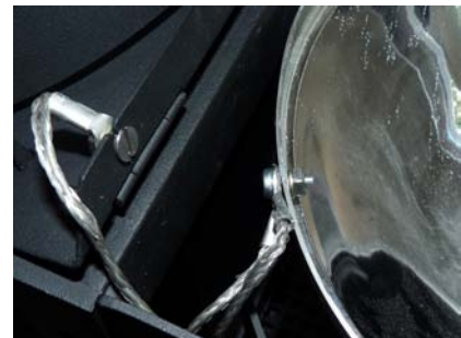
Earth connection to reflectors
