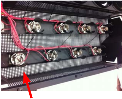
Cable routing (1 & 6 by the right side, others left side)
